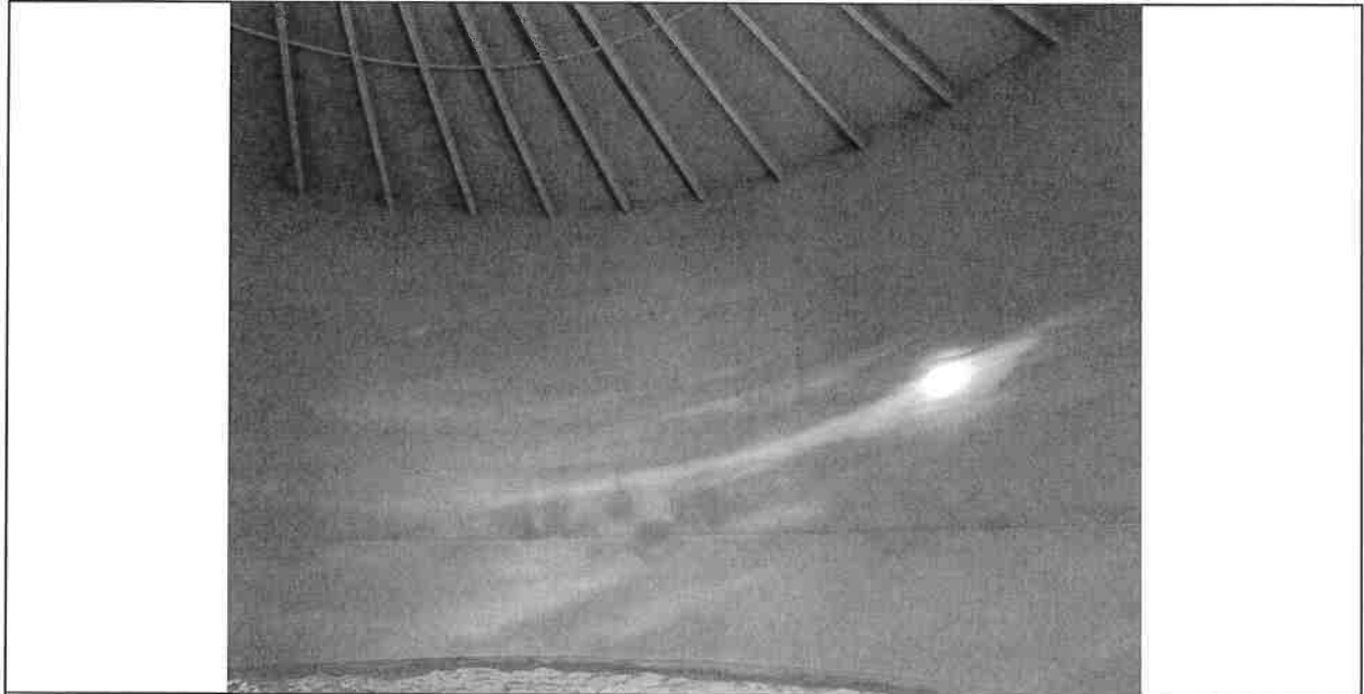
Interior Completed abrasive blasting meeting and exceeding specified SSPC SP10 "Near White" metal abrasive blast.
