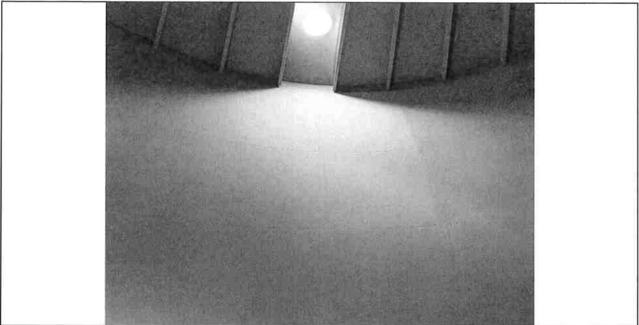
Interior Completed abrasive blasting meeting and exceeding specified SSPC SP10 "Near White" metal abrasive blast.
